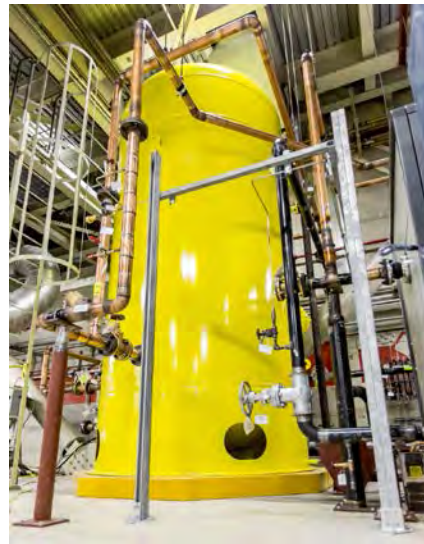
Breathing Air Installation
